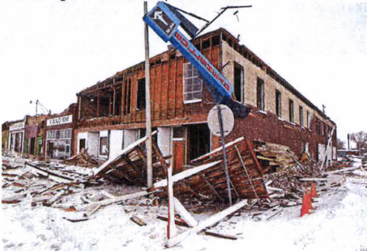
Picture Credit: Damage in the historic district of downtown Wells, Nevada, as a 6.0 earthquake at 6:16 am PST today. (Tom Smart, Deseret Morning News)
