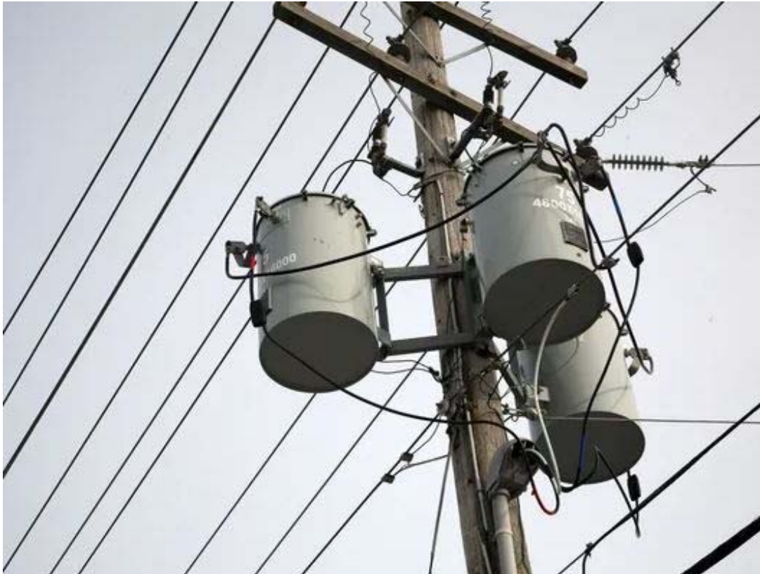
Utility pole with power lines and transformers.
