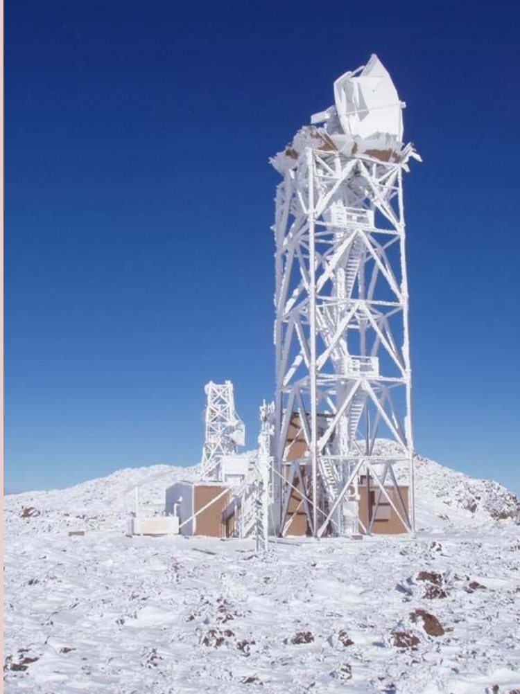
Figure 4-4 NWS Reno Radar Damage from Wind (December 2008)
