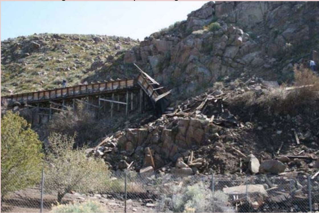
Rock fall damage to water flume
