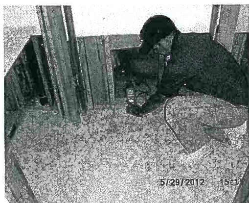
Moisture reading from under the tub
