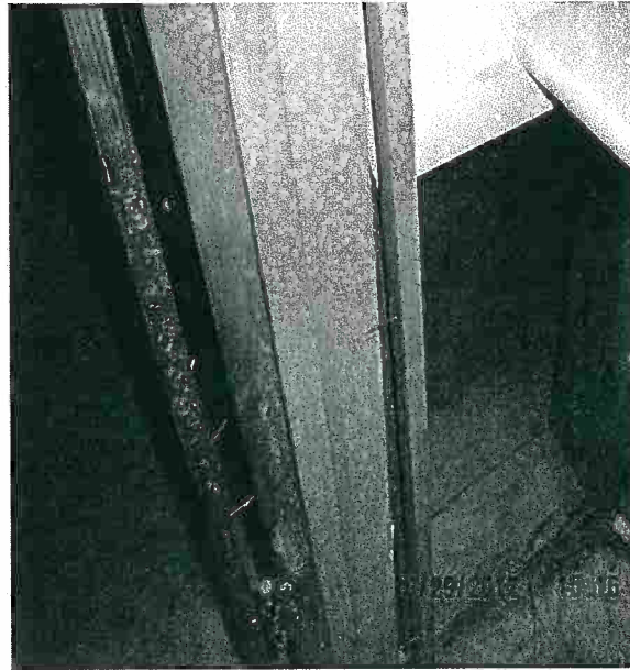
Damage caused to the jambs and casings as a result of chemicals and cleaning solutions used by the prior mitigation service.
