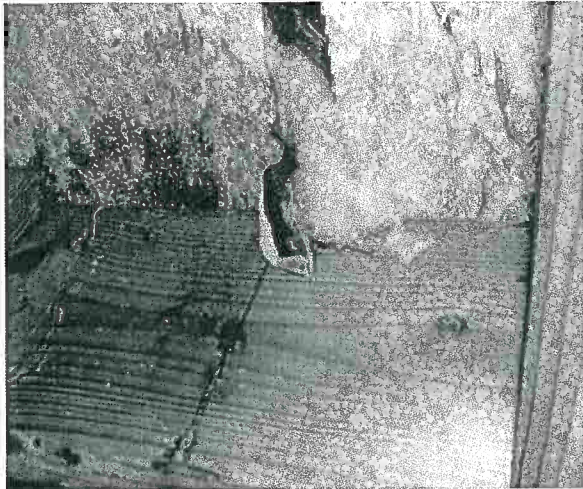
Mold Growth under the dressing room
