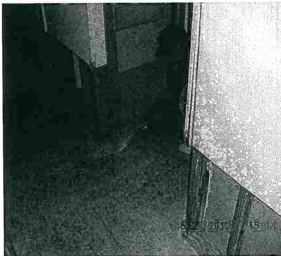
Particle board under the tile floor Hall bath
