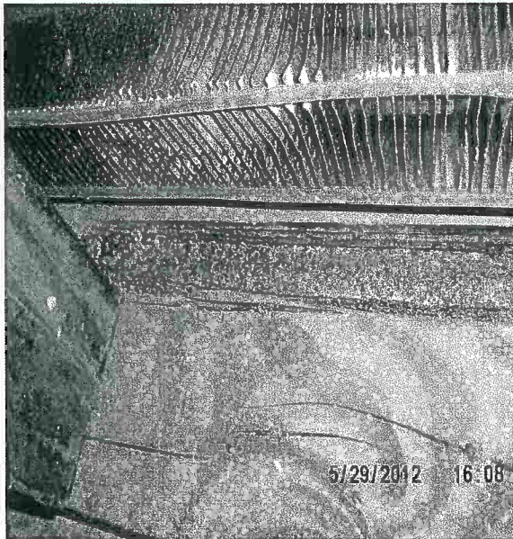
Damage caused to the hydronic heating radiator fins. Typical throughout the affected area.
